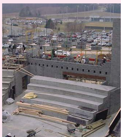
Construction of an 850-seat auditorium at the high school provided an opportunity to test rigid foam insulation placed in service nearly 10 years before.
